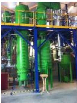
Pilot plant for biomass gasification
