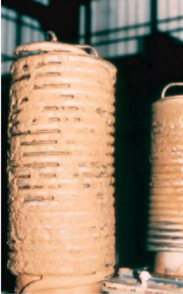
Fig. 2 Heat exchanger of a pump, protected by a biodegradable corrosion inhibitor, after 6 months of operation. The corrosion inhibitor is completely degraded and causes massive biofouling
